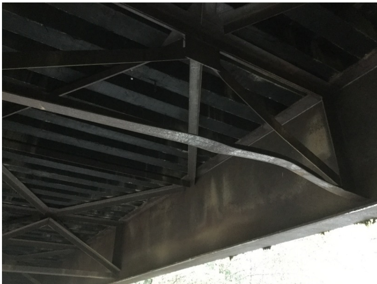
Bottom chord on 2nd diaphragm on right bank distorted
